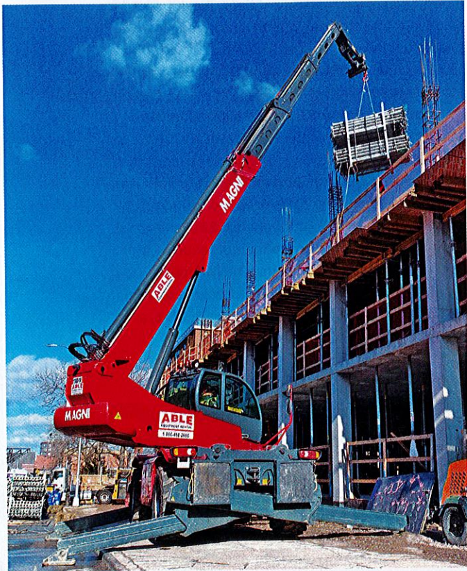
A Magni telehandler, part of Able Equipment Rental's fleet, on a jobsite last year. Photo by Able Equipment Rental
